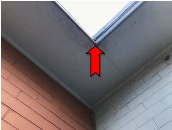
Photo 1. Exterior, throughout, eaves – asbestos-containing fibre cement sheeting.
